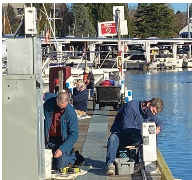
Vessel Electrical Safety Committee upgrades dock three terminals
