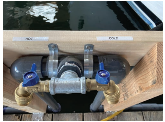
Water Works on Docks Two & Three thanks to the Docks Committee Crew
